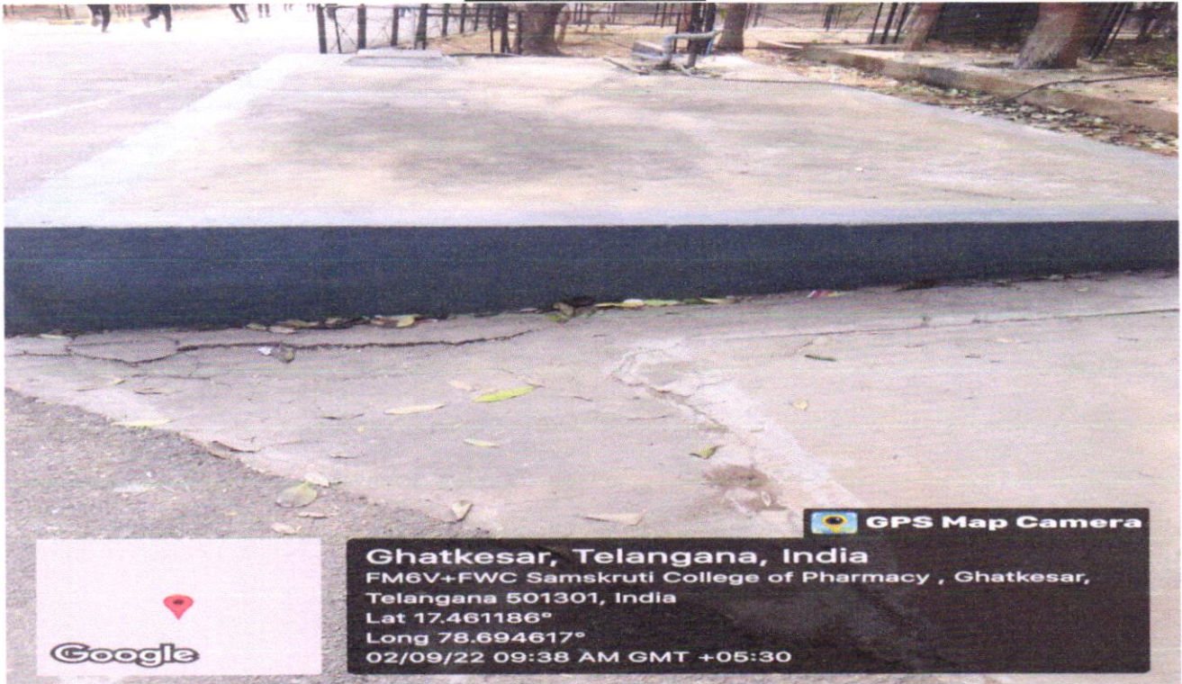
Common Water tank
